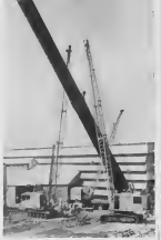
In the first picture workmen are removing the scaffolding built up around the stack so crane hooks could be attached.
